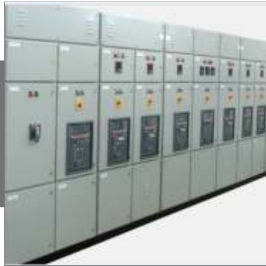
POWER CONTROL CENTER
