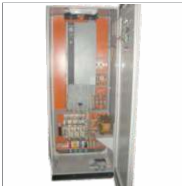
VFD CONTROL PANEL
