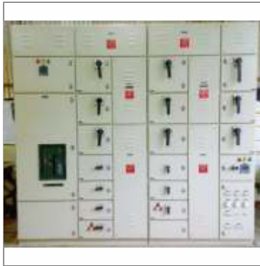
POWER DISTRIBUTION BOARD
